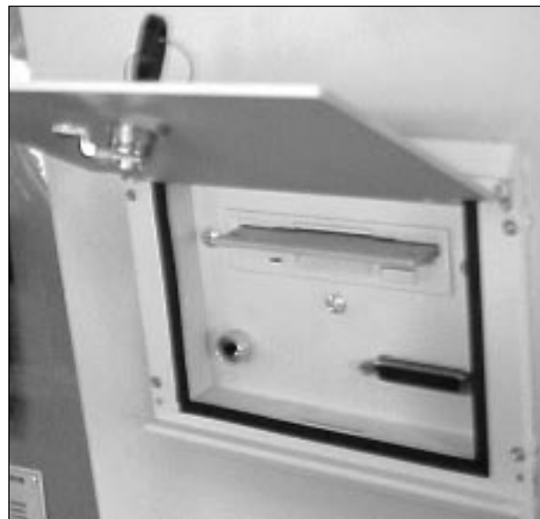
Figure 1-19. Floppy Drive and RS232 outlet (with cover) on left side of electrical cabinet.
